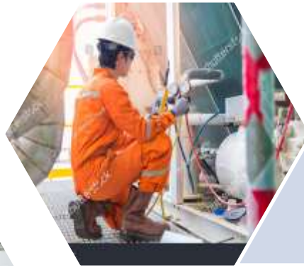
Pipe Line services
